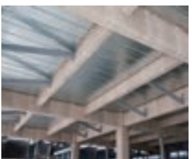
Wrap-type rock wool fire-proofing covering materials
